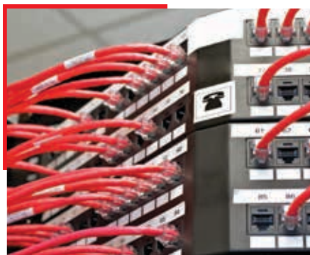
Networking of Active Components (Switches, Routers & Firewalls etc.)
